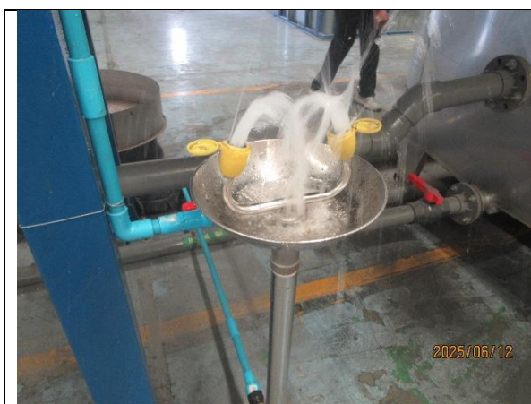
Eye washing facility
