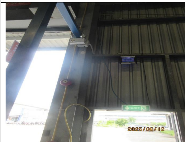
Safety exit and emergency light
