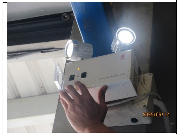
Emergency light testing
